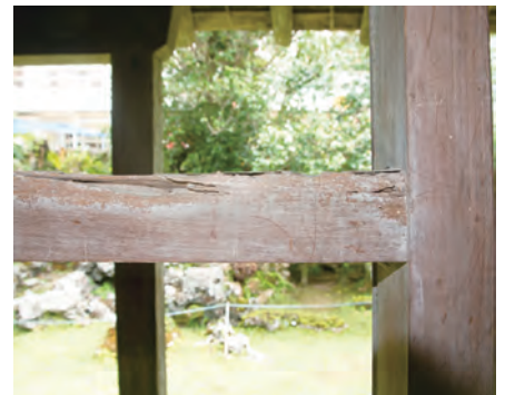
Figure 14. Current condition. The doorframe for hawk paintings b and c. Termite damage remains in places. Photograph collection of Chie Kyan. Permission of Ishigaki City Board of Education.
