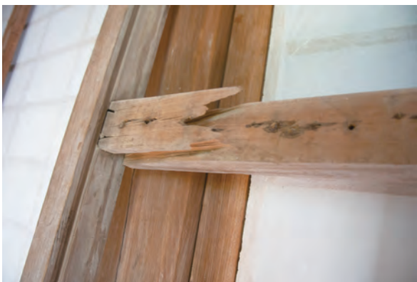
Figure 15. Current condition. The doorframe for hawk paintings b and c. The iron nails have expanded due to rusting, and the wooden frame has been damaged. Photograph collection of Chie Kyan. Permission of Ishigaki City Board of Education.
